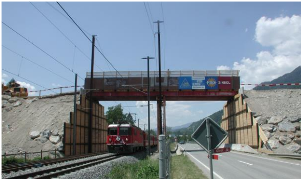
Figure 6, Temporary GRS in Switzerland using locally Fill Material and Soldier Beam Method
